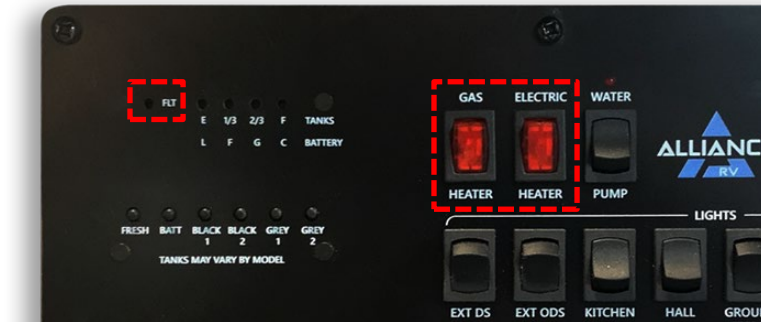
Figure 135. The water heater power switches on the main Monitor Panel. The FLT light is highlighted on the left. These are also shown in Figure 111A and D.
