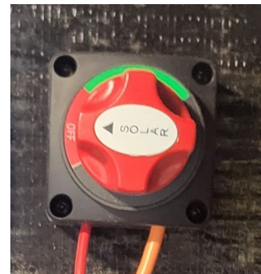
Figure 83. Solar disconnect switch.
