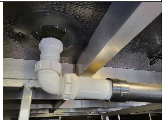
Figure 132. Waterless p-trap under a shower location.
