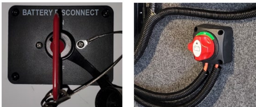
Figure 61. Battery disconnect switches. Original style, left, and new style, right.
