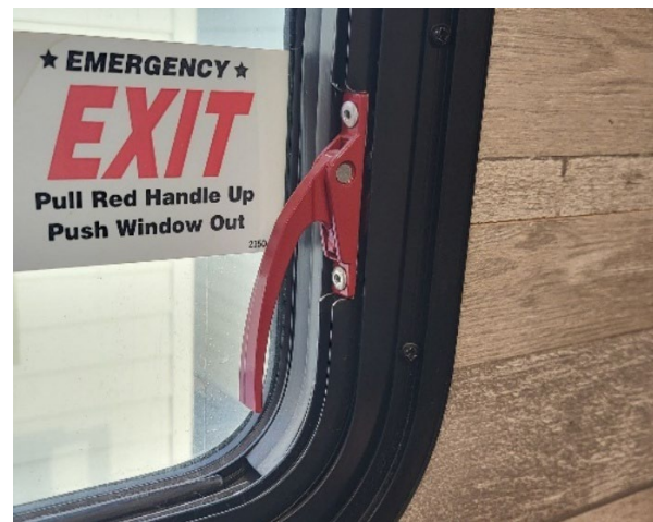
Figure 24. Pull-Lever style latch on an emergency exit. Pull the lever out, away from base, to disengage latch. Push window out.
