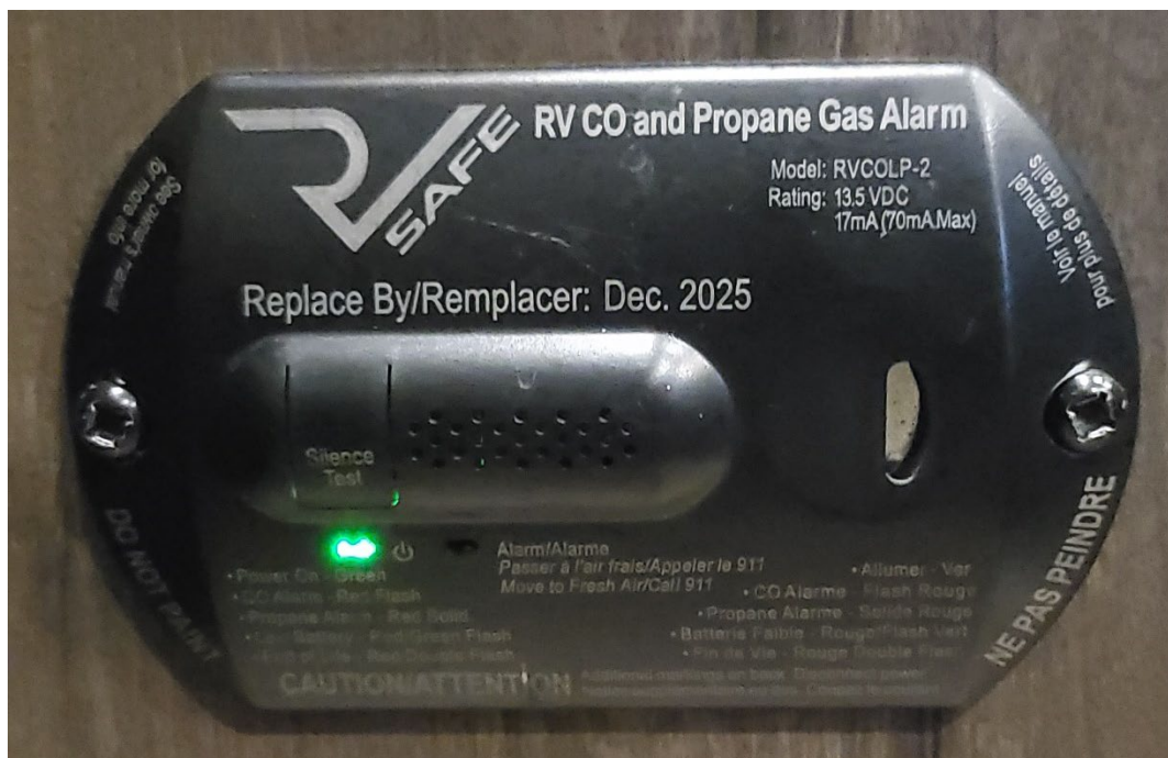
Figure 27. Wall mounted Carbon Monoxide (CO) and Propane alarm. These will be mounted near floor level, usually near stairs.
